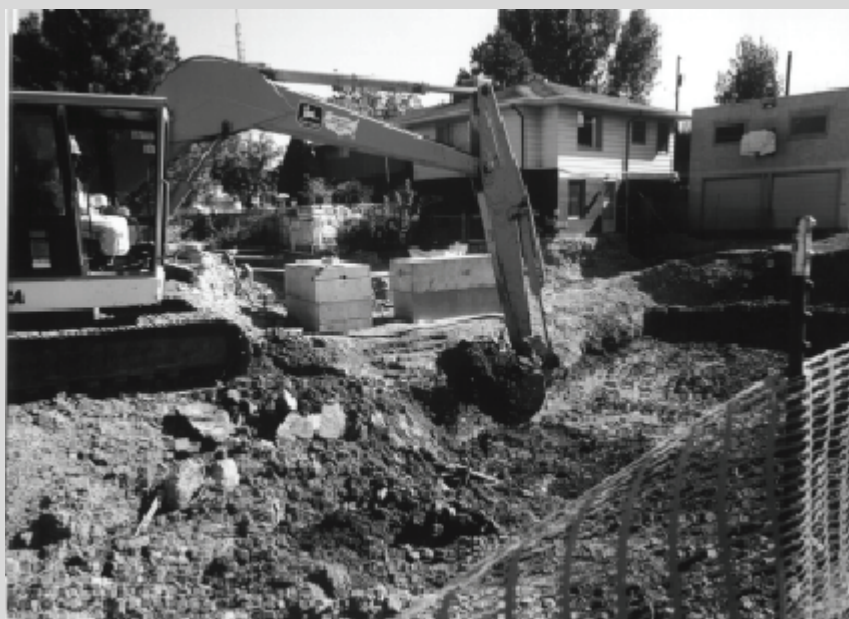
FIGURE 7.2 Excavation of uranium mill tailings from a residential septic system, Grand Junction, Colorado, 1993. SOURCE: U.S. DOE Office of Environmental Management.
